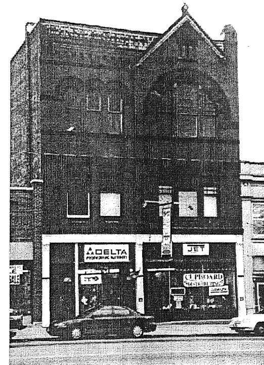
Visually Clattered Storefront as a Result of Many Different Signs Placed Along the Glass Front. The Base of the Building is Visually Separated from the Upper Parts.
