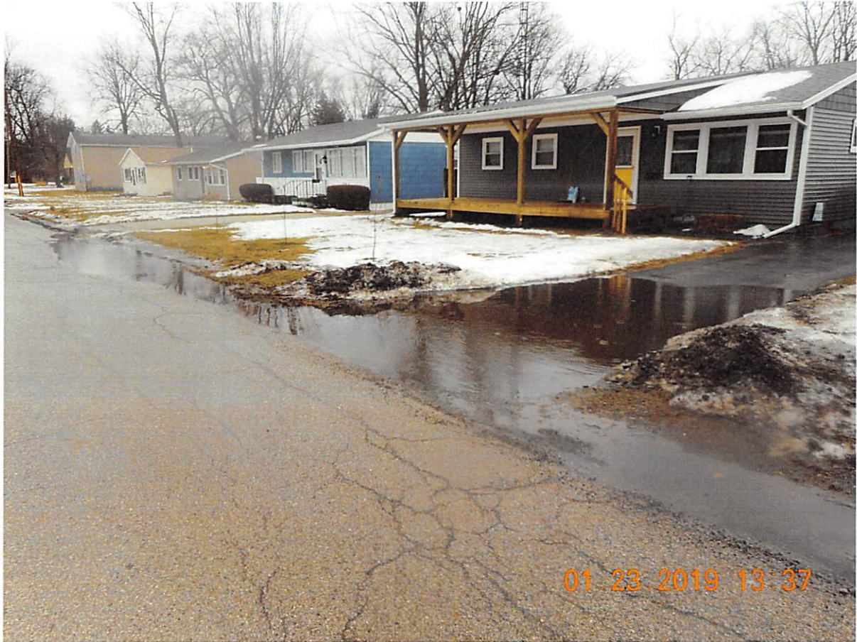
Existing South High Street (looking north) between Thompson Street and Hovey Street
