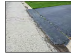
EXAMPLE: Filled Gutter
