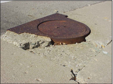
METAL OR OTHER PLATES, COVERS, OR GRATINGS THAT ARE NOT FLUSH (1/2 INCH OR MORE VERTICAL DIFFERENCE) WITH THE ADJOINING SIDEWALK SURFACE, ARE STRUCTURALLY UNSAFE, OR CAUSE A NUISANCE DUE TO SLIPPERY SURFACES ETC.
