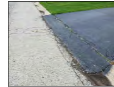
EXAMPLE: Filled Gutter
