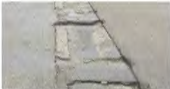
EXAMPLE: Large Holes in Surface
